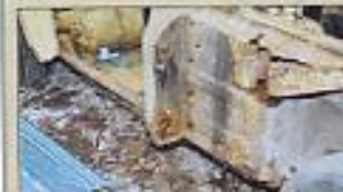
Corrosion hidden by the outer sills and front wings.
